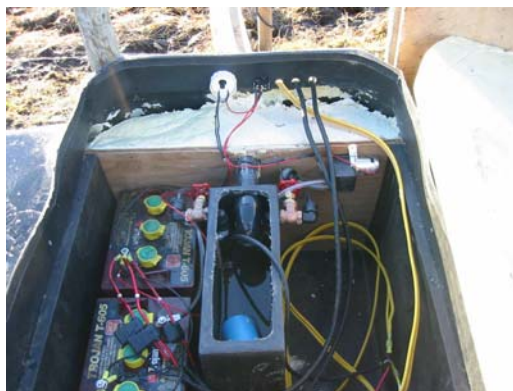
Two 6 volt batteries, connected via cable to each other and to the two 105 watt solar panels.
