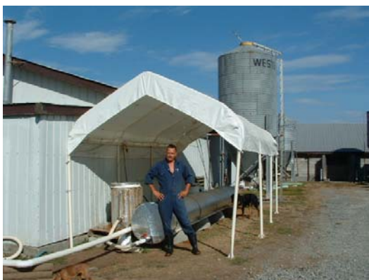
A pilot scale plug flow digester was installed at John Doppenburg's hog farm.
